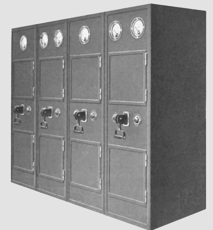
Switch cabinet distribution after 7 years of operation
